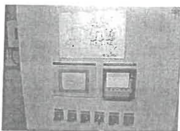
Figure 10: Control panels and flow chart
